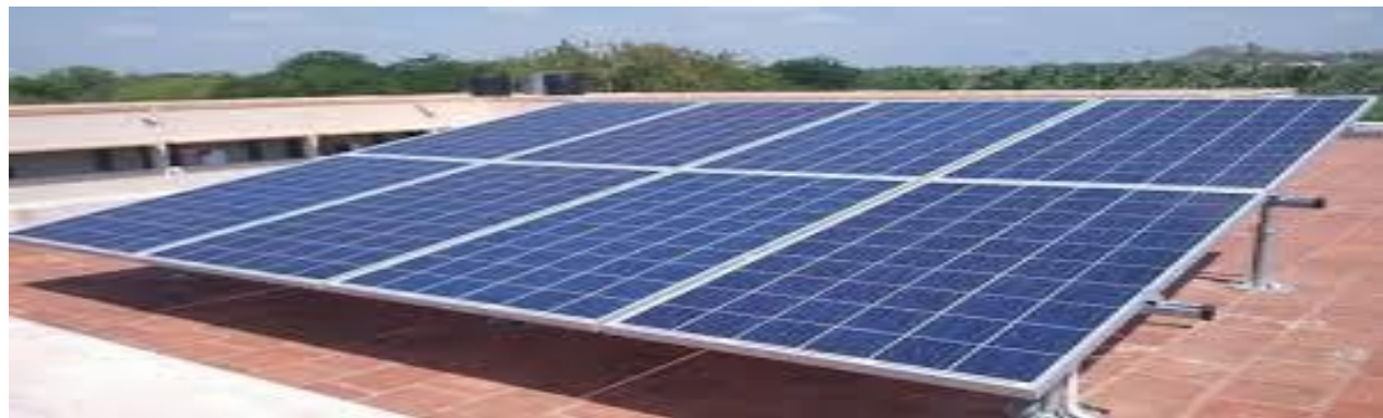
1250 kW capacity Solar installed on Building roofs of all 4 Units
