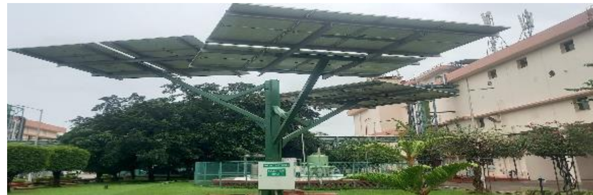
12 kW Solar Tree installed in Factory Premise
